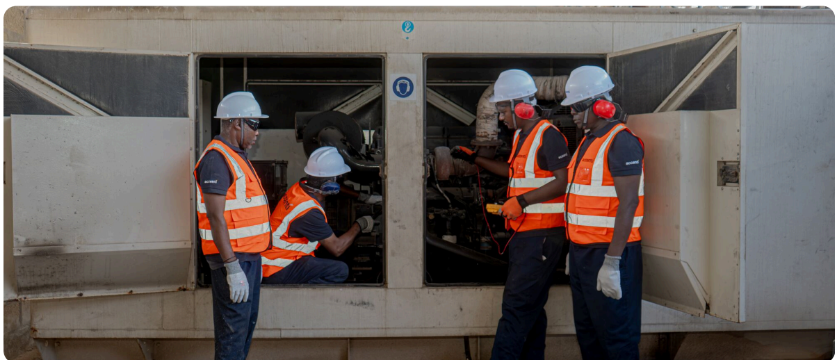
— Generator servicing with hearing, eye and hand protection in place.
